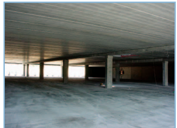
Precast columns and beams used to complement the long span Hollow Core planks.
